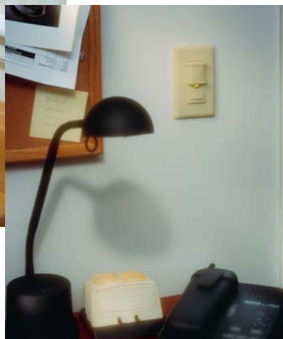
Motion sensors save energy automatically.
