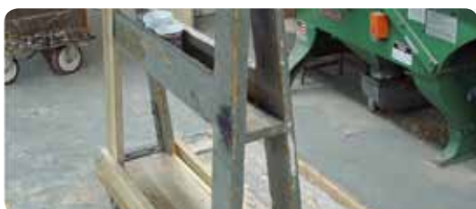
Wood - Splinters and rots
