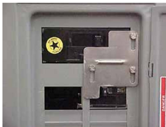
Generator Interlock Kit (In use)
