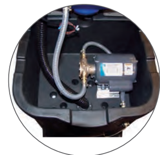
Discharge pump located in equipment bay rather than recovery tank
