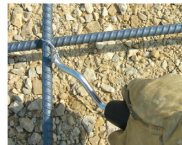
Typical TWTT installation
